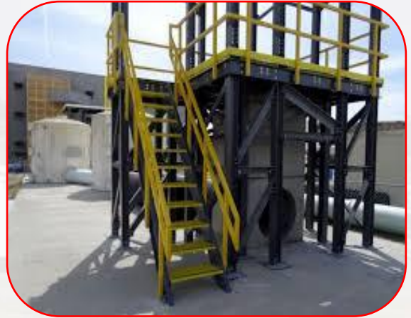
Industrial platforms and walkways
